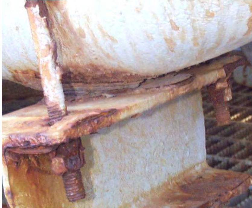
Figure 7. Advanced Crevice Corrosion
