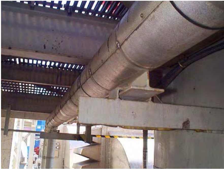
Figure 5. Typical Welded Pipe Support
