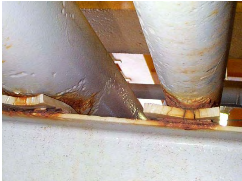
Figure 8. Rubber Pads Accelerate Crevice Corrosion
