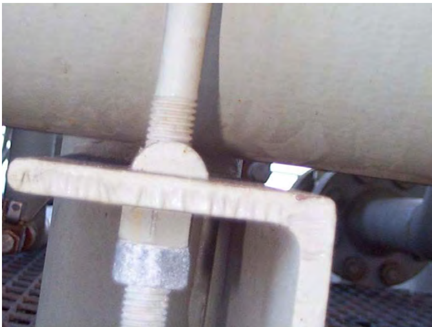
Figure 10. The Half-Round Pipe Support Interface
