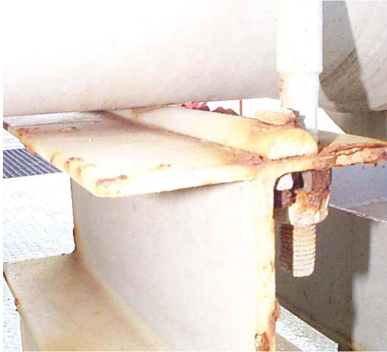
Figure 15. Rod in Place Under Pig Launch Barrel – 13 Years
