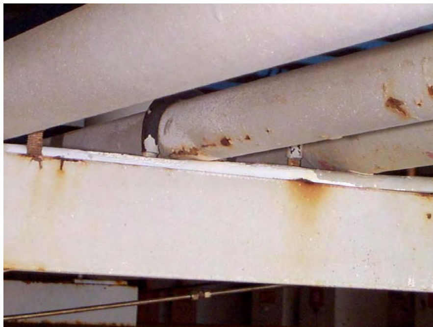
Figure 14. Beam Dressing Supports After 13 Years Offshore
