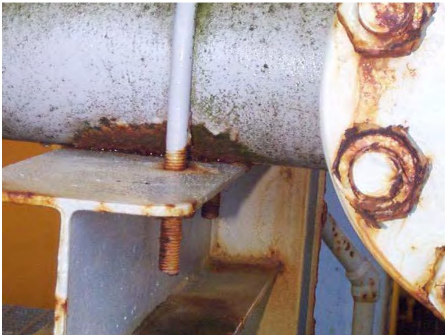
Figure 6. Progressive Paint Undercut Away From Initiation Site
