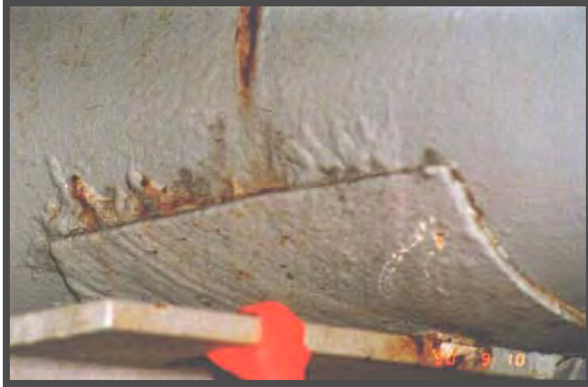
Figure 9. Fiberglass Contoured Pads Still Risk Crevice Corrosion
