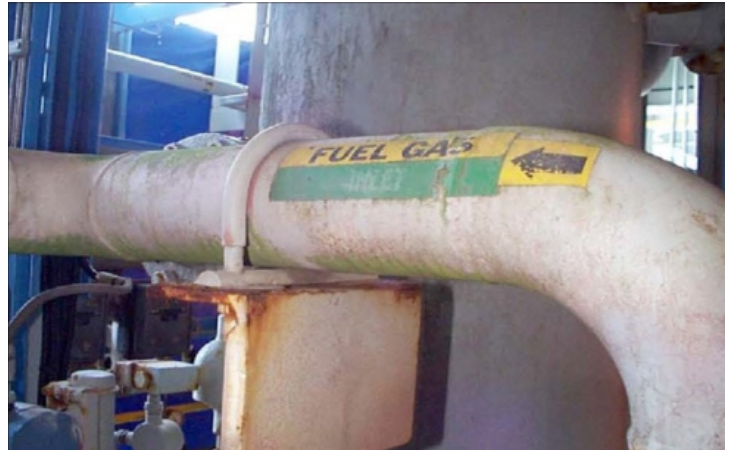
CONSTANTLY WET This fuel gas line is always wet (the green coloration is mold) and the beam paint system has failed, but no corrosion has occurred at the pipe support..
