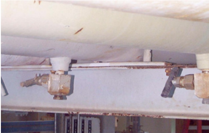
HOLDING UP WELL I-Rod was used to dress beams beneath multiple pipes. There's no crevice corrosion.
