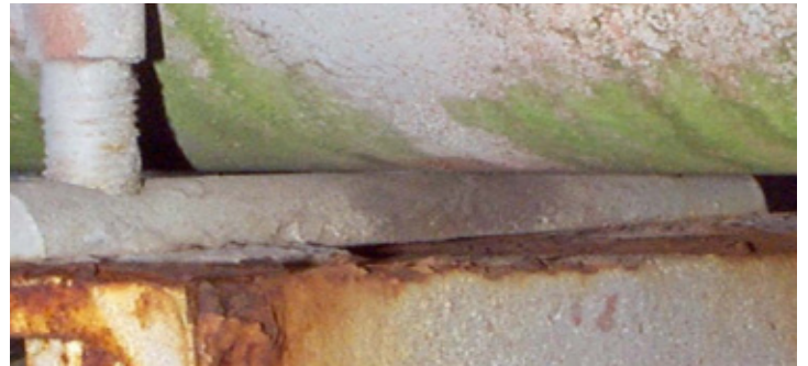
A CLOSER LOOK Here's a closer look at the pipe support shown in the top photo above...
