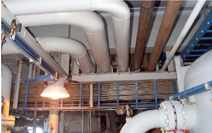
WELL-DRESSED SUPPORTS More beam dressing on a typical pipe rack. This is 1" I-Rod.
