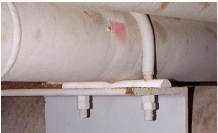
TEST OF TIME This Nu-Bolt never corroded, but has picked up a coat of paint over the years.
