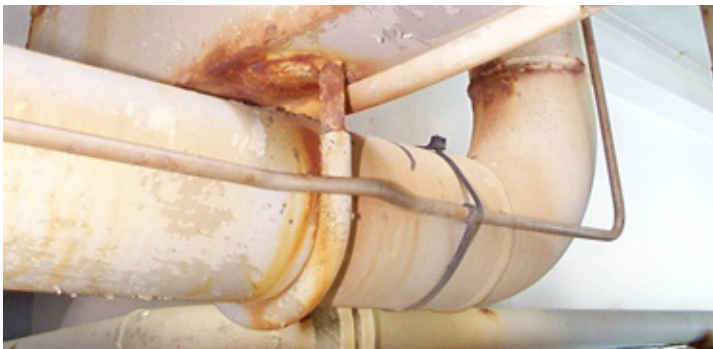
LOOKS WORSE THAN IT IS Another instance where the paint has failed but there's no crevice corrosion.
