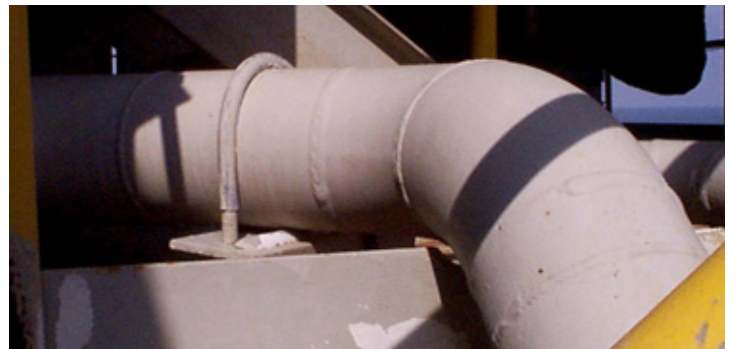
STILL IN GOOD SHAPE The pipe remains well-preserved despite the harsh offshore environment.
