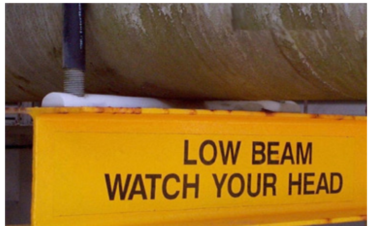
SAVED BY I-ROD A close-up of the support at left shows why the wet pipe remained in good condition.
