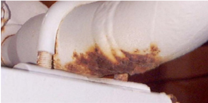
DRIP POINT (ELL CORROSION). Crevice corrosion at the support is less than on girth weld. Without I-Rod, this would have been a failure point.
