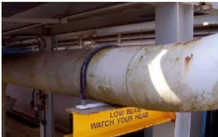
LOW BEAM, HIGH RISK Another pipe that stays wet, as evidenced by the mold and mildew on its surface.
