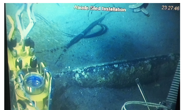
RETROCLAMP ESTABLISHES ELECTRICAL CONTINUITY BETWEEN THE SLEDS AND THE STRUCTURE. THIS CLAMP IS FITTED A FIXED MONITORING SYSTEM.
