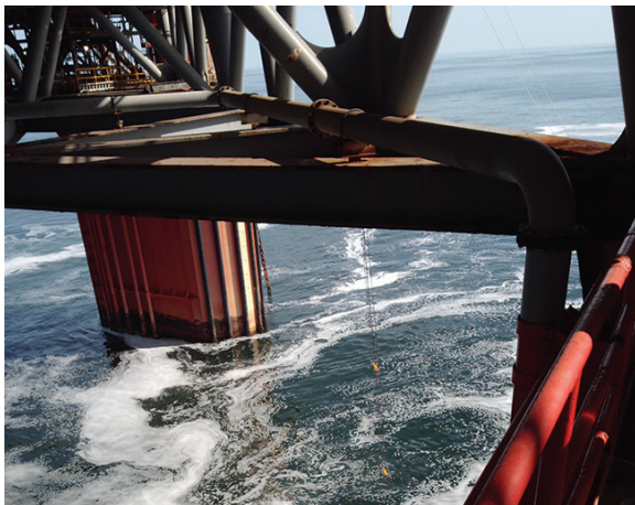
WHERE DAT CP? After a decade in service, the original CP was close to completely failing.
