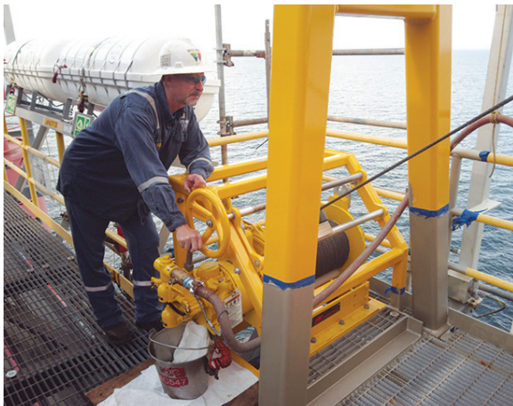
SUSPENDED AND RECOVERABLE ANODES. A winch system allows recovery of the suspended anodes.
