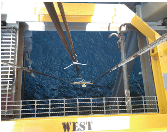
TETHERED NEAR THE SEA FLOOR The anodes are tethered in place to minimize damage from turbulent water.
