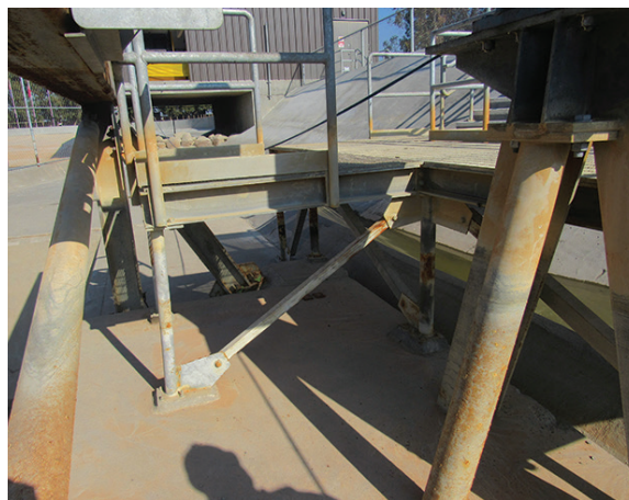
TREATED WATER NOT SUCH A TREAT Chemicals that were used to keep the water clear may have hastened corrosion.
