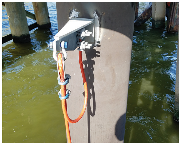
SAVING THE DOLPHINS RetroLink™ anode strings were used on the individual dolphins.
