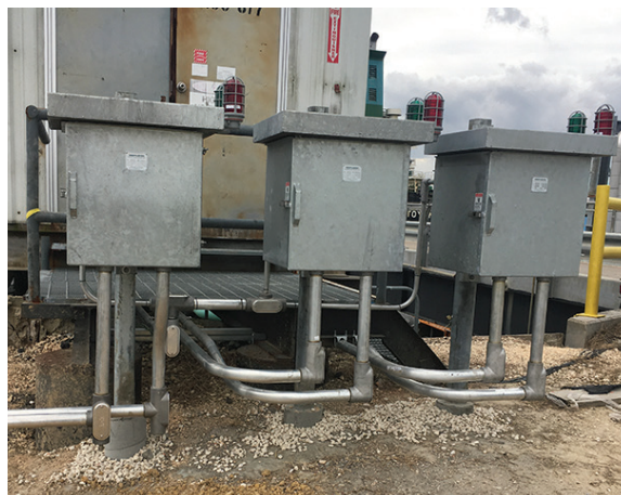
TRANSFORMER/RECTIFIERS One unit powers one ICCP sled; a total of 15 were installed.
