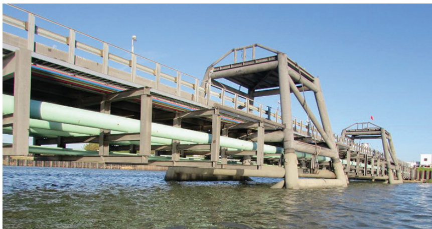
PROVIDING CONTINUITY Over 100 continuity brackets were added and multiple sheet piles were welded together to provide electrical continuity.
