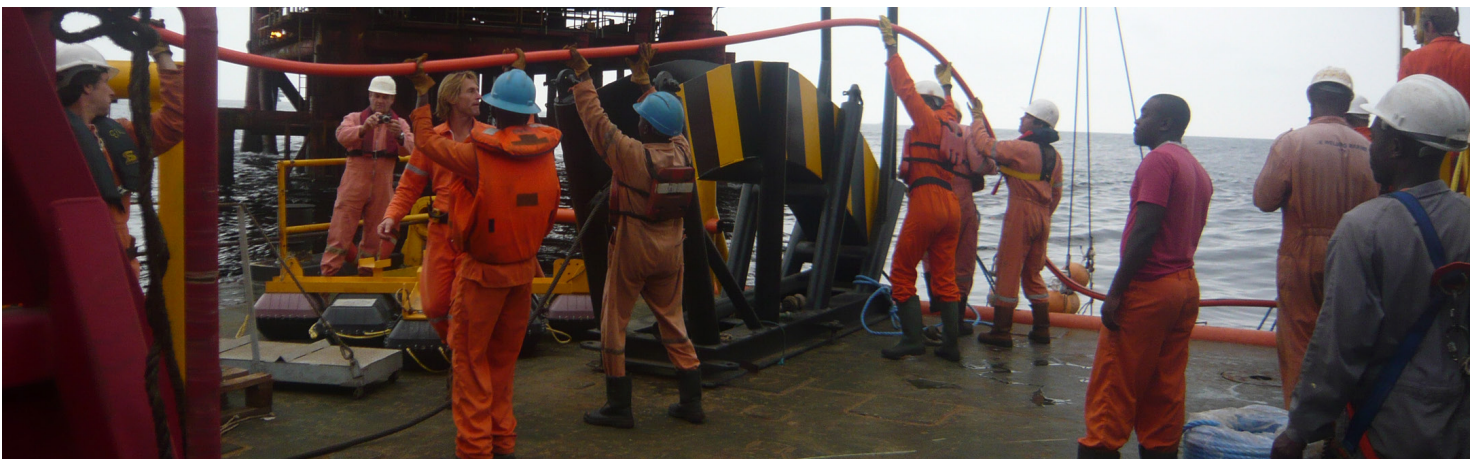
ALMOST DONE Once the RetroBuoy™ is on the seabed, an ROV will complete the installation.
