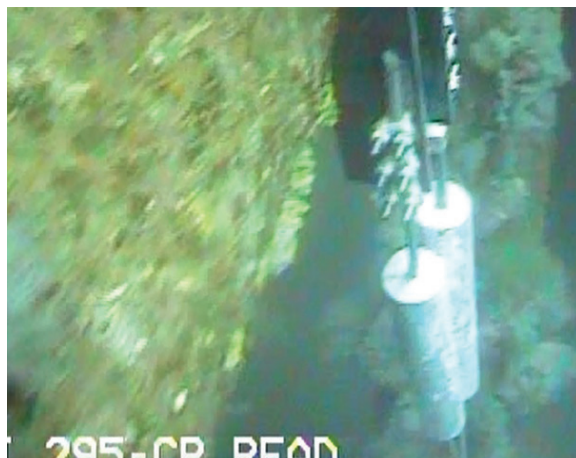
THE VIEW FROM BELOW The RetroLinks™ hang from a subsea clamp.
