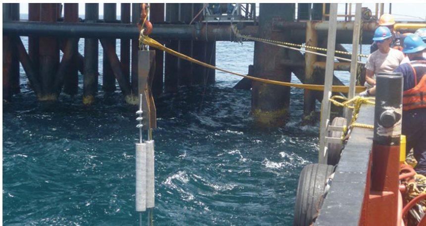
DOWN THEY GO The RetroLink™ anode strings are lowered into place by workers on the work boat.
