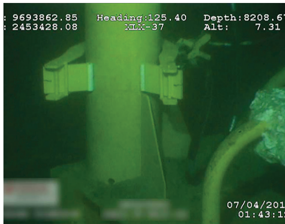
CONTINUITY ESTABLISHED RetroClamp™ end of bonding jumper connected to the PLET’s tubular receptacle.
