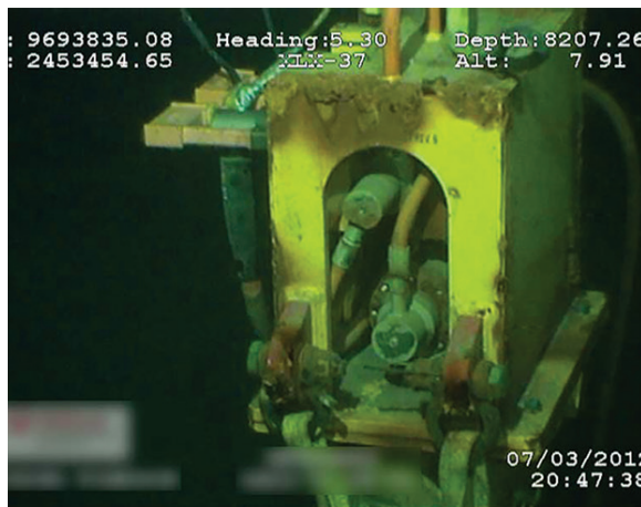
MINI-GATEWAY END VIEW The mini-gateway showed active corrosion from lack of cathodic protection.
