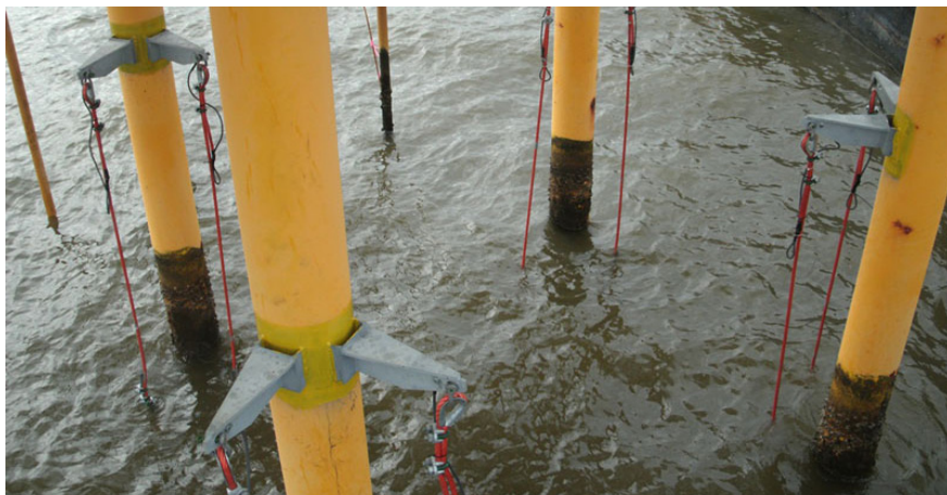
LOTS OF STRINGS ATTACHED Anode strings are suspended from stand-offs welded to the risers.
