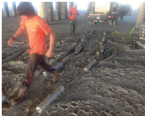
RAPID INSTALLATION RetroLinks™ had been stored beneath the pier to expedite deployment.
