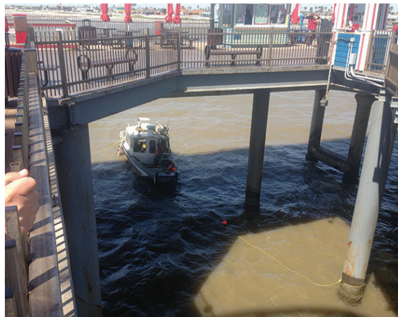
CP IN TOW Once attached, the RetroLinks™ were towed away from the pier and positioned.
