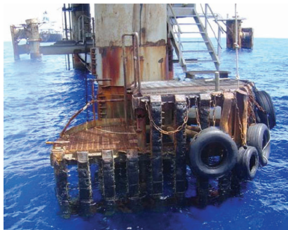
LOADING TERMINAL The existing anodes on this terminal had begun to fail to protect the structure.
