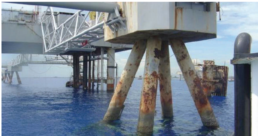
TIME FOR RETROLINKS™ When the impressed-current system began to fail, the owners opted for a sacrificial anode CP system.
