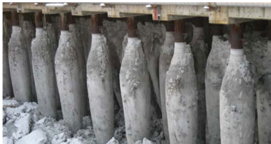
DEEP FREEZE When the wharf freezes and thaws each winter, the piles and anodes are completely encased in ice.
