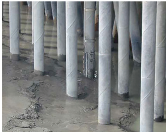
ROUGH NEIGHBORHOOD All previous pile anodes failed in the brutal freeze-and-thaw environment.
