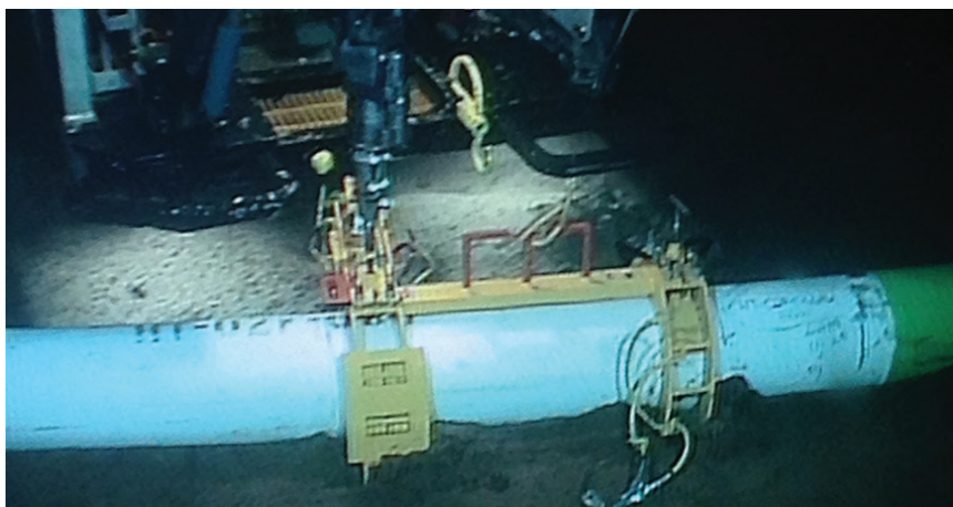
CLAMPED DOWN Here's the dual clamp assembly after installation on a flow line. The contact tip provides connection when tightened.
