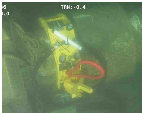
WEST CLAMP The RetroClamp™ was able to squeeze into this spot just West of the flange.
