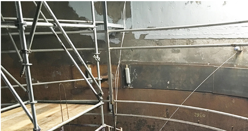
FLUSH-MOUNTED ANODES In addition to the new anodes, a CP monitoring system was installed using V-String™ reference electrodes.
