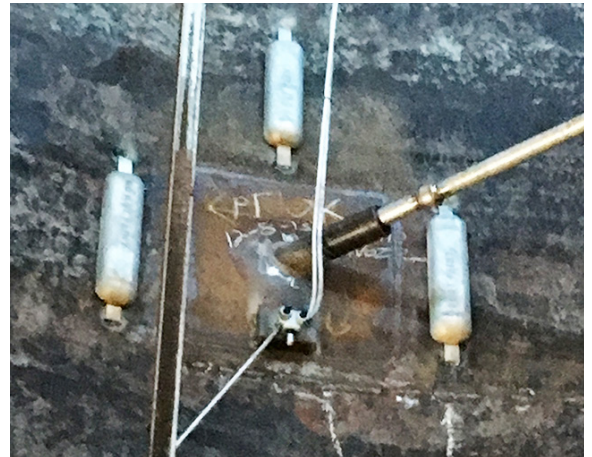
12 ANODES INSTALLED The anodes were placed around all four heating coil inlet and outlet nozzles.
