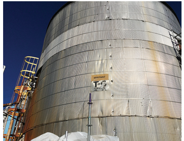
THE PROUD RECIPIENT Storage tank T-6 received a new set of anodes and a new lease on life.
