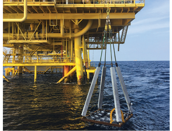
PODS FOR THE PLATFORM, SLEDS FOR THE PIPELINE Retrofitting the platforms took 20 RetroPods™.
