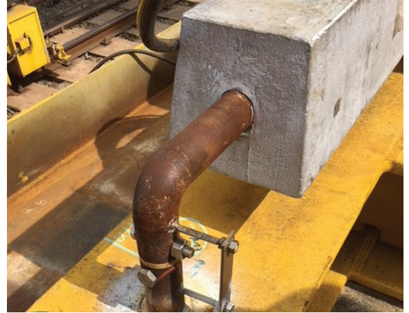
MA-1 MONITORED ANODE ON THE SPOOL CONNECTION ASSEMBLY The MA-1 will track anode performance and consumption.
