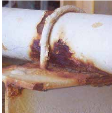
Above, the result of crevice corrosion on a pipe. Trapped moisture has caused substantial wall loss that could result in catastrophic failure.
