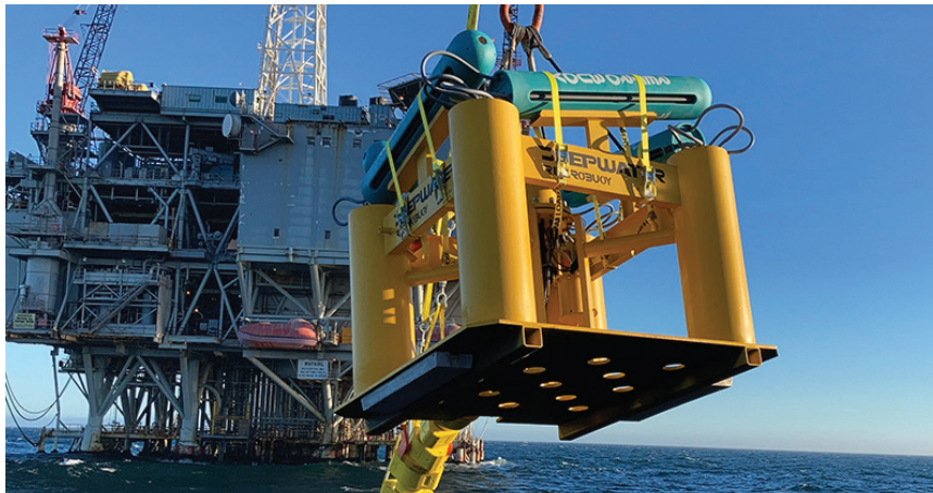
ONE DOWN, TWENTY TO GO Positioning a RetroBuoy™ for deployment in the largest offshore ICCP retrofit ever done in a single campaign.
