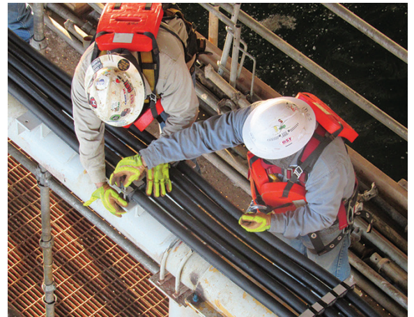
SAVING MONEY WHILE SAVING STRUCTURES Still-functional elements of the existing ICCP system were re-used to cut costs.
