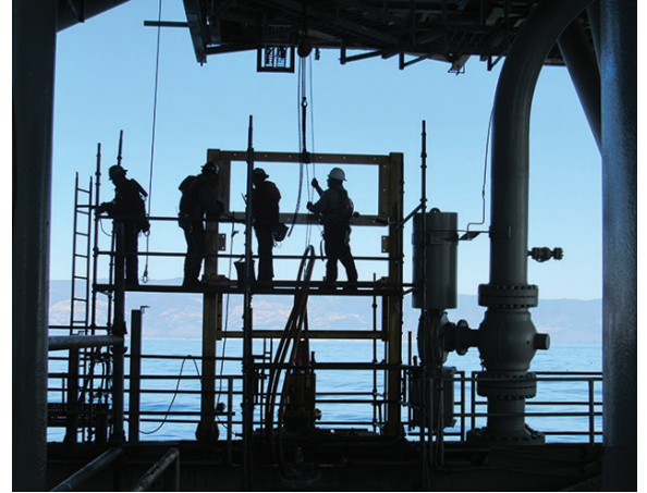
OUT OF HARM'S WAY Junction boxes were raised an extra 11 feet to prevent flooding in high seas.
