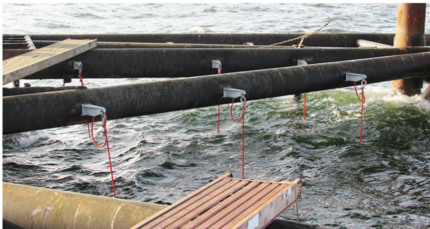
PLENTY OF PROTECTION The CP retrofit involved attaching 44 RetroLink™ anode strings that were longer than usual.
