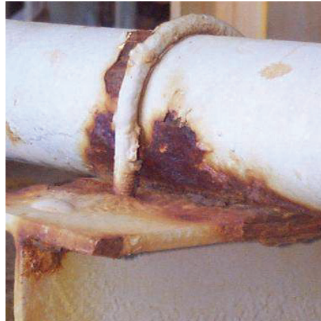
Above, the result of crevice corrosion on a pipe. Trapped moisture has caused substantial wall loss that could result in catastrophic failure.
