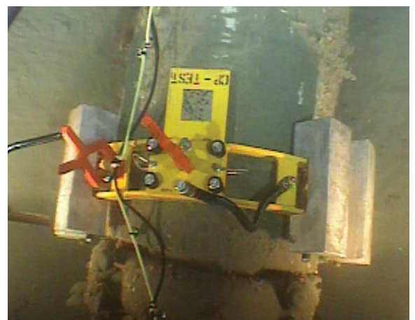
FAST INSTALLATION Most of these clamps were installed in less than an hour each.
